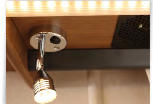
Low voltage lighting
