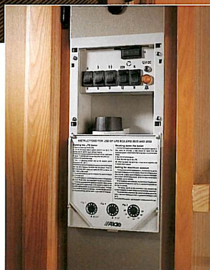
The Alde Swedish central heating system provides interior comfort and domestic hot water from both gas and electric sources.
