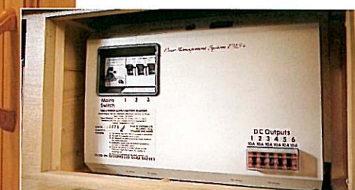
C. E. C. Power management system
