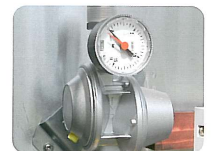
Fitted gas regulator
