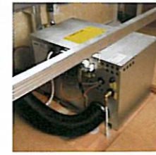
Alde heating/hot water system
