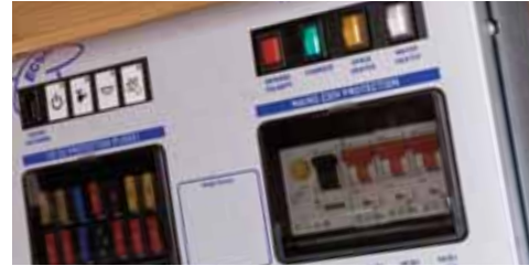
Charger/transformer and RCD unit
