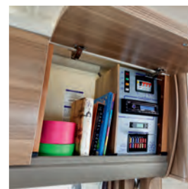
^ Locker mounted eye level power supply unit and power management for easy access
