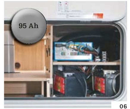
06 On-board HVAC&S systems: AGM living area battery with 95 Ah capacity positioned next to heater
